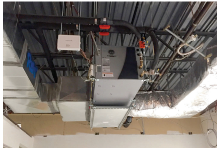
GSHP Installed Above Suspended Ceiling. This GSHP supports multiple heating and cooling zones.
