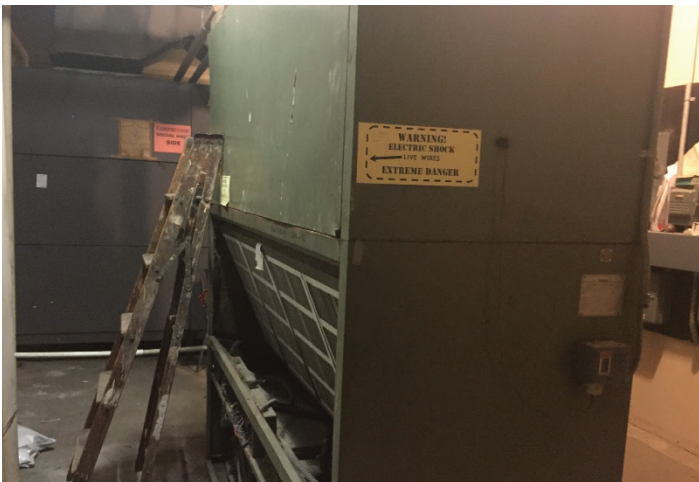
Antiquated Equipment Before Replacement
