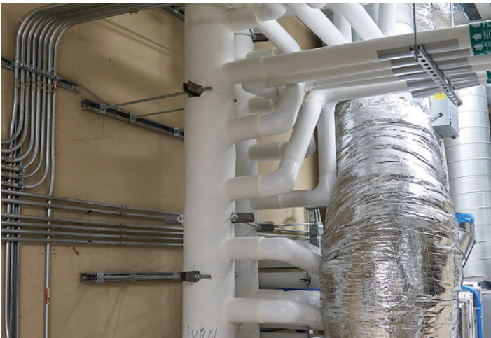
Building Geothermal Piping
