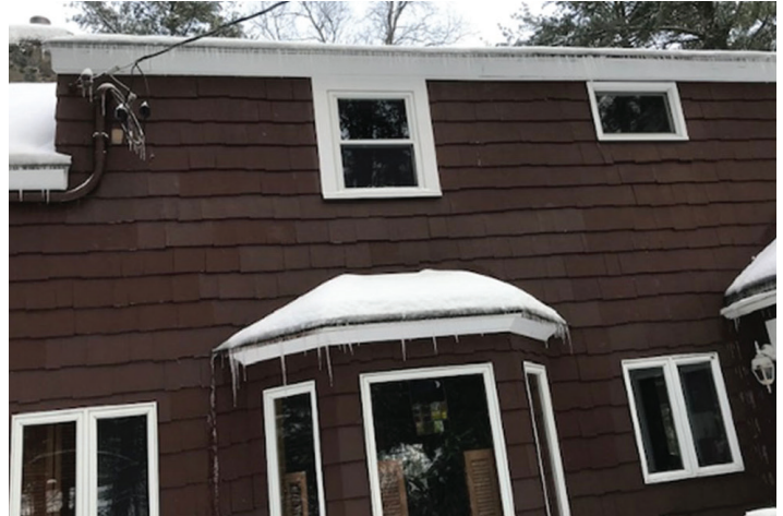
Ice Issue Mitigated by Insulation/GSHP Install
